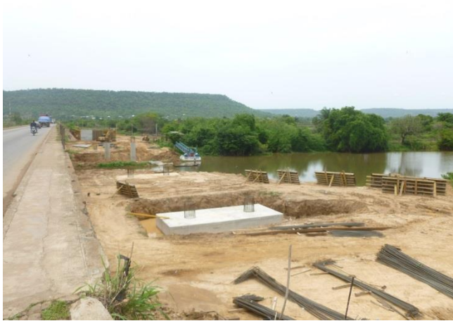
Plate 3: Bridge construction for the 2 nd lane of the Lokoja-Abuja highway near Kotonkarfe.
