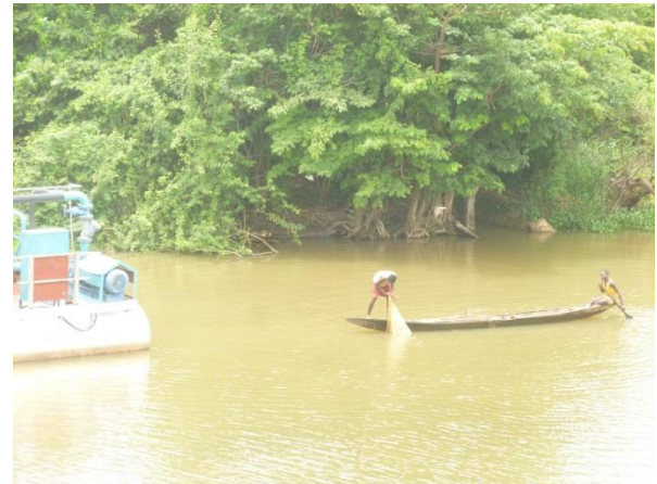
Plate 4: Increased water turbidity caused by run-off from earth work during bridge construction
